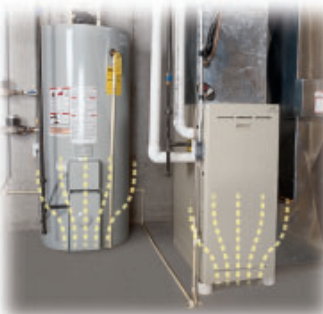
Regular maintenance of equipment can keep you safe from CO.
